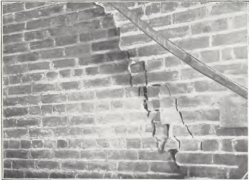
B. EFFECT OF SEVERE SHAKING ON WELL-BONDED BRICKWORK FILLED WITH GOOD MORTAR, TOWER OF UNION FERRY BUILDING.
